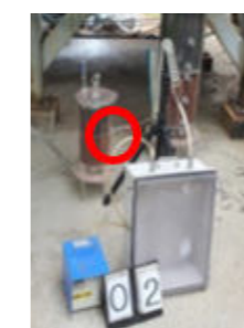
1 st deodorization bed
