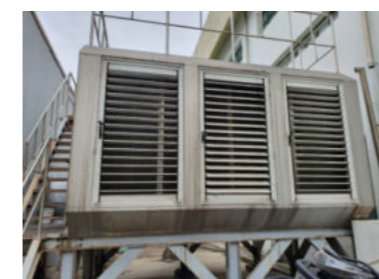
Existing odor removal equipment (4.7m 3 * 3part = 14.1 m 3 )
